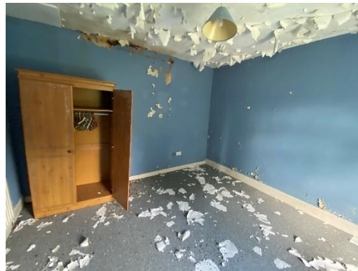
Plate 4-6 Internal room on the second floor showing widespread peeling paint and scattered bat droppings.
