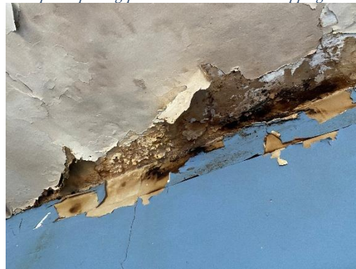
Plate 4-8 Staining on the ceiling of an upper-storey bedroom, consistent with bat occupancy.
