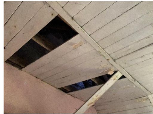
Plate 4-10 Internal view of Structure 8 showing accessible attic space via broken ceiling planks.
