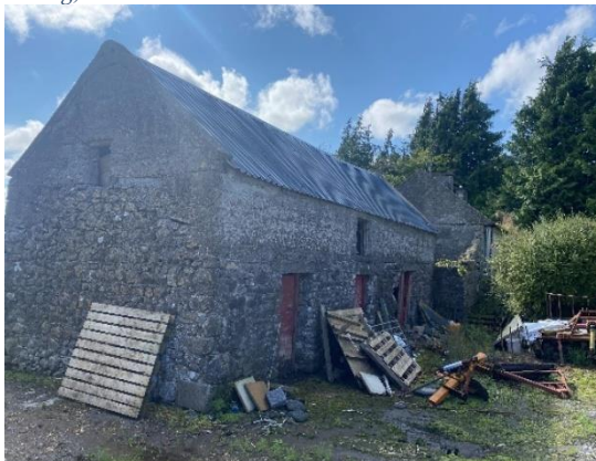
Plate 4-15 Exterior view of Structure 10 - crevices in the wall which may provide roosting potential.
