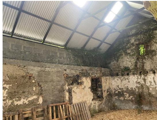
Plate 4-14 Interior of the farm shed showing exposed roofing, with minor crevices between bricks and concrete.
