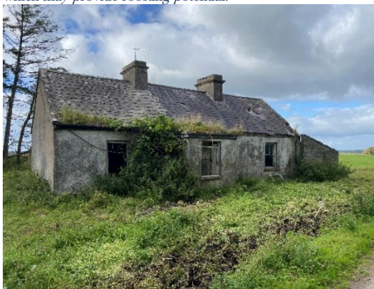
Plate 4-17 External view of the storage farmhouse Structure 12 showing lifted slates and general condition of the roof.
