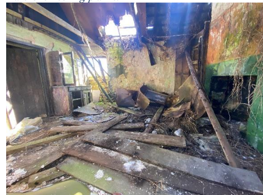
Plate 4-12 Internal view of Structure 6, showing fallen planks and lack of underfelt, indicative of limited shelter for roosting bats.
