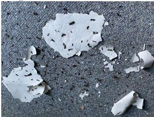
Plate 4-7 Close-up view of bat droppings on the floor in an upper-storey bedroom.
