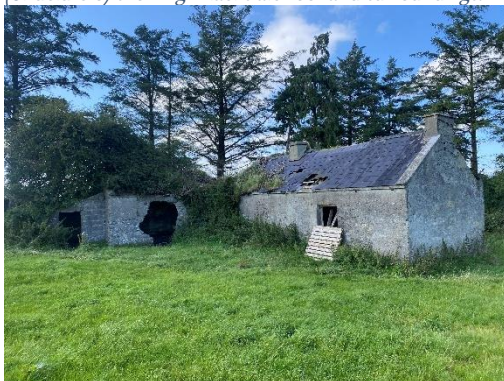
Plate 4-11 External view of the derelict building (Structure 6), showing broken roof slates, and surrounding habitat.
